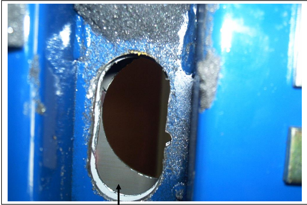
Hole from engine compartment side.
